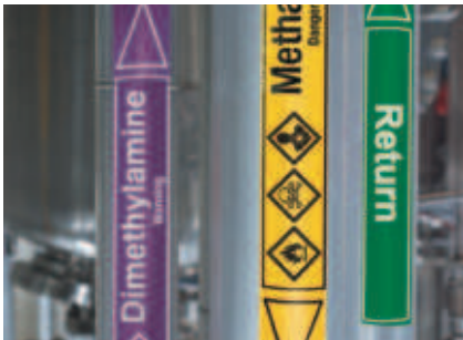
Pipe & valve marking
