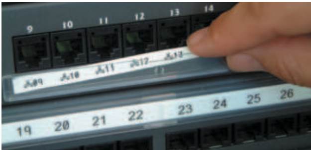
Punch block & patch panel labels
